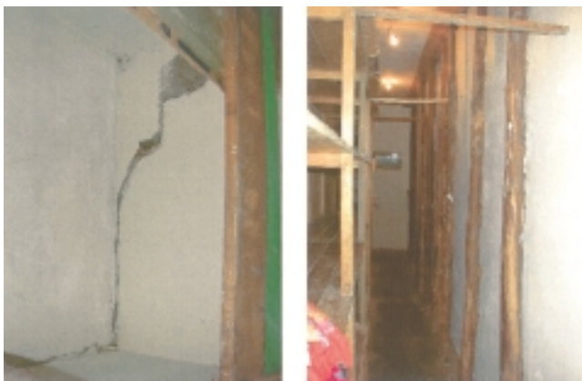
Fig.13 Cracks progressing in the wall and their temporal reinforcement by timbers inside the Luggage Check beneath the open cafe of Machu Picchu Sanctuary Lobge
