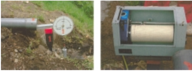
Fig. 8 Two types of extensometers installed in Machu Picchu citadel. Left: Simplified type extensometer (#1 in Fig. 9) which was developed for monitoring of active / potential landslides in Machu Picchu citadel. Right: Self-recording type extensometers (S-1 in Fig. 9).
