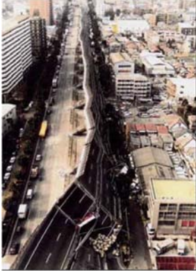
Collapse of highway piers
